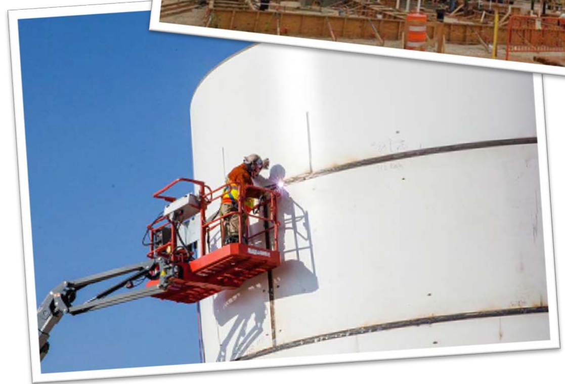
Construction of the new Fire Water Tanks for the Fire Water Loop System
